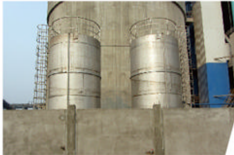
华新襄阳公司脱硝现场液氨储罐 Huaxin Xiangyang plant denitration plant
