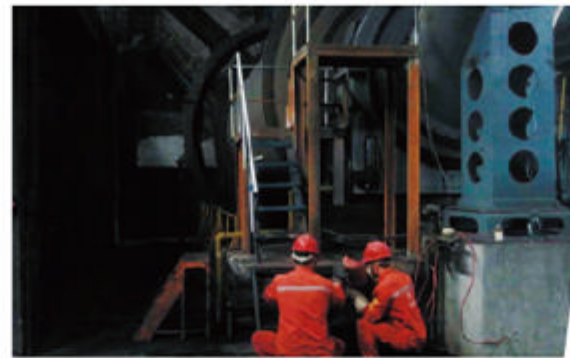
岗位工自主整改K5煤磨操作平台 Workers autonomously corrected K5 coal mill operation platform.
