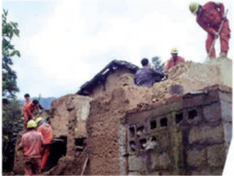
志愿者为灾区群众修补房屋 / Volunteers repair houses for people in disaster area
